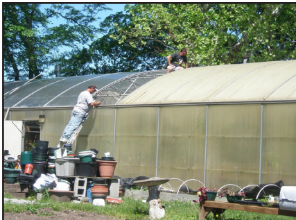
Workers replace the roof of the Sims Greenhouse. The old Plexiglas roof was cracked and was blocking the sunlight.
